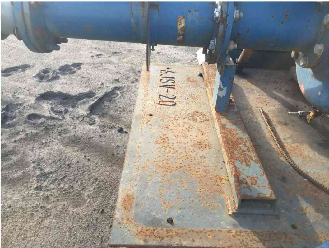
Figure 4 – Photographs of Unit 2 Slurry Pond Pump
