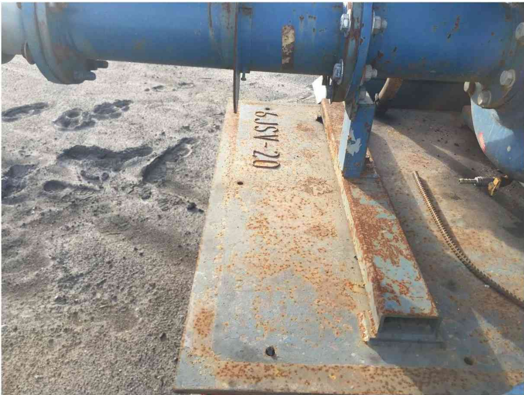
Figure 4 – Photographs of Unit 2 Slurry Pond Pump
